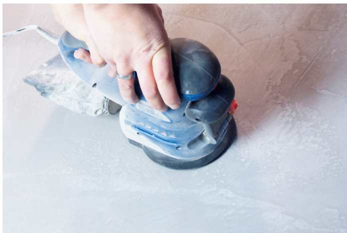
24 hours after applying the 2nd coat, sand with a hand sander the surface with a disc of 80 then 120.
