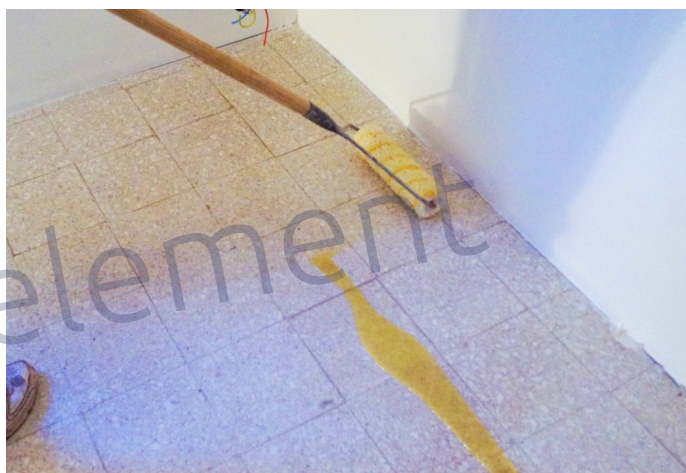
Apply the epoxy resin using a medium pile roller. Work in strip of 1 m not forgetting any part of the tiling.
